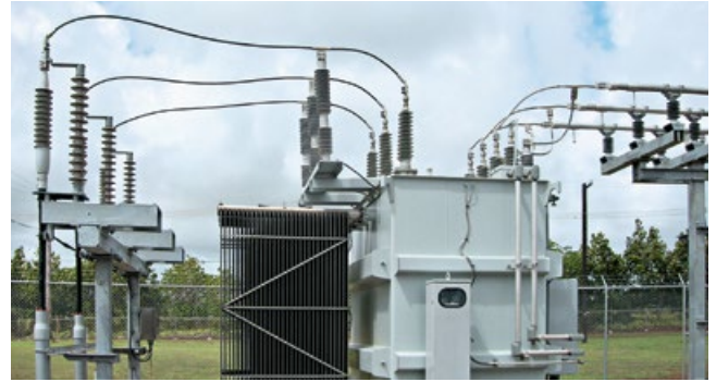
Oil- and gas-free solid insulation: Outside the substation, the IXOSIL terminations connect the cable with the transformer.
