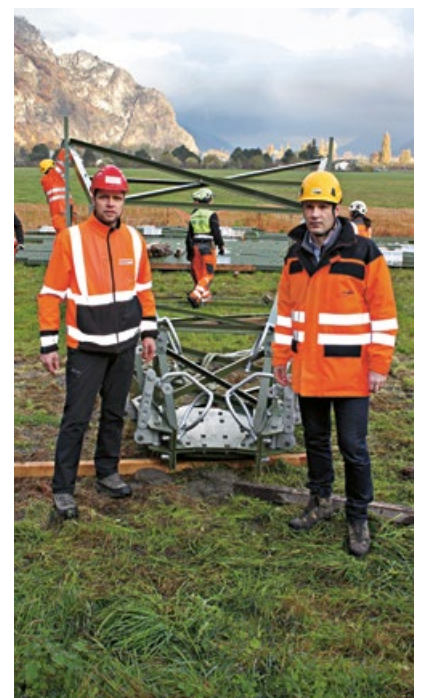
Pre-assembly: Helmut Burgener (l.), PFISTERER project manager, and Michael Eichenberger (r.), CEO of Eduard Steiner, inspect a pre-assembled crossarm with pre-installed PFISTERER string fittings, from the tower suspension to the arc-rings.
