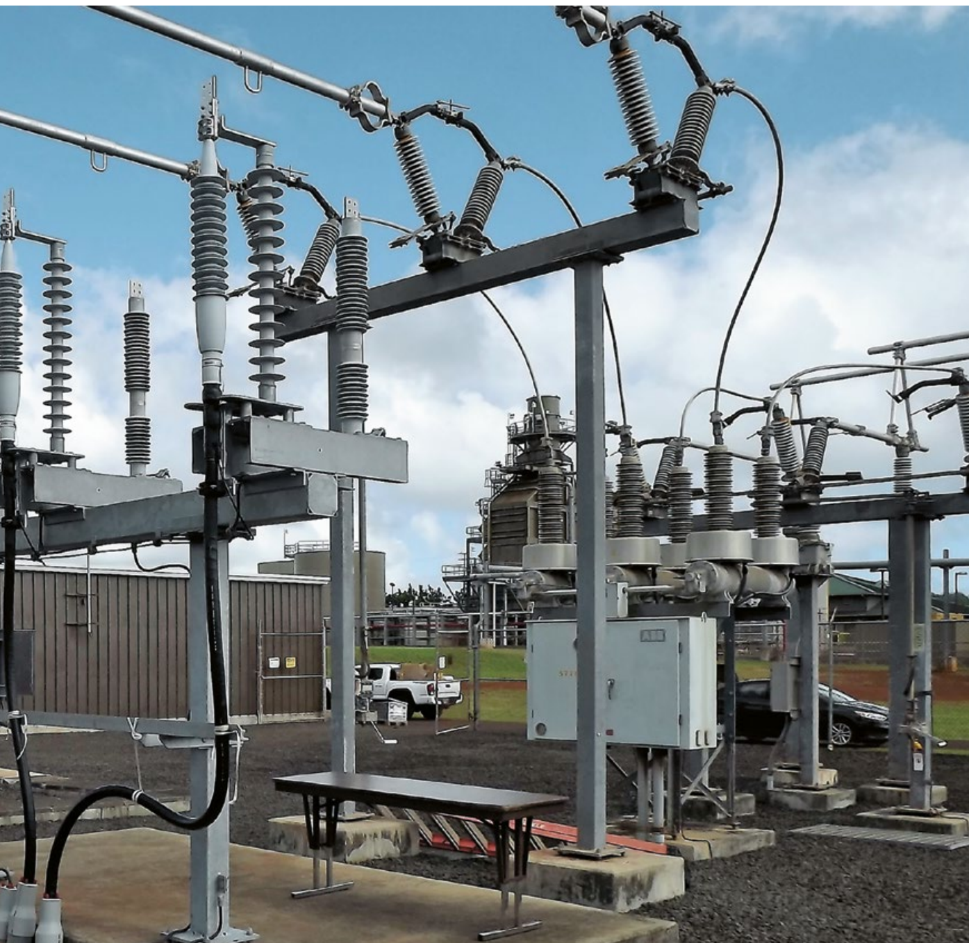
Reliably safe and resource-preserving power supply: Inside the substation, three self-supporting dry cable terminations are connected with the overhead power line via the tap-changer mechanism.
