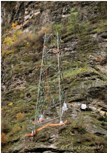
High performance at altitude: Installation engineers assemble the elements of tower 124, which is anchored into an extremely steep rock face.
