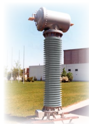
245 kV Current Transformer manufactured in 1975
