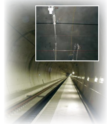
High Speed Track in the Swiss Loetschberg Tunnel
