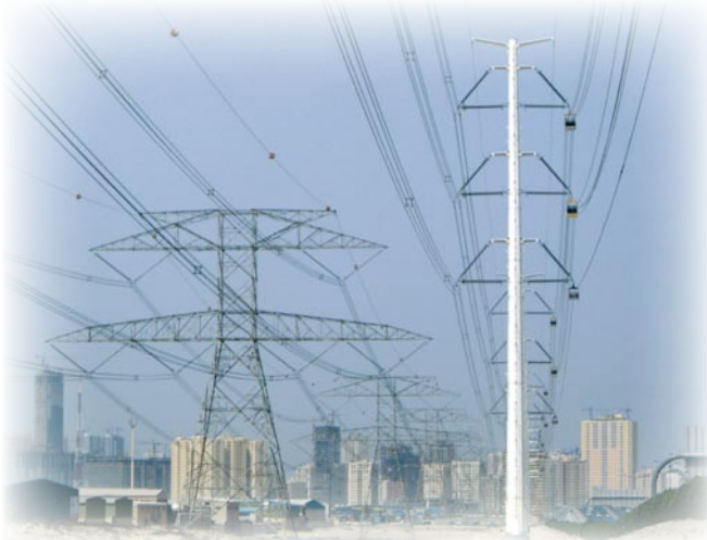
DEWA's 420 kV Compact Line
