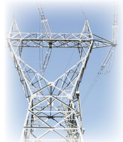
ATEL's 420 kV Line with 500 kN Force Rating
