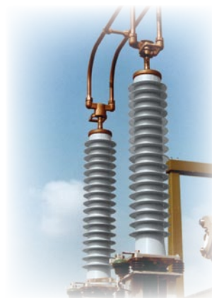
123 kV Cable Termination installed in 1975
