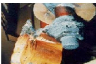
Small cause, big damage: Improper contacts disable expensive operating equipment.
