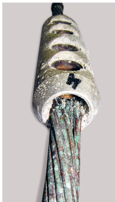
Figure 8: Conductors and connectors after ten weeks of salt resistance testing according to IEC 60068-2-52
