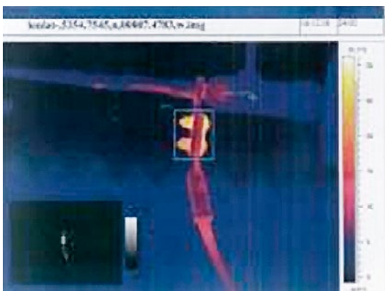
Figure 1: An analysis of the thermal image shows that the bolts are by far the hottest area in the tested terminal set-up. This means that the current flows through the bolts rather than the contacts—a precursor to contact failure.
