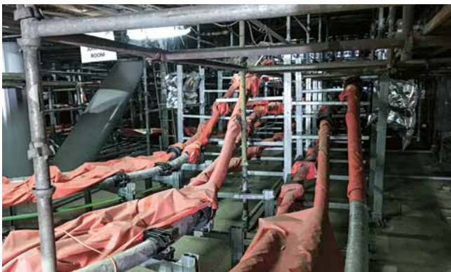
HV cable systems inside the platform. The cables are covered to protect them from heat and dust.
