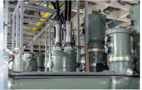
Turnkey cable systems for DolWin gamma. Extremely flexible Feltflex cables run over several platform levels and connect to the gasinsulated switchgear with CONNEX.
