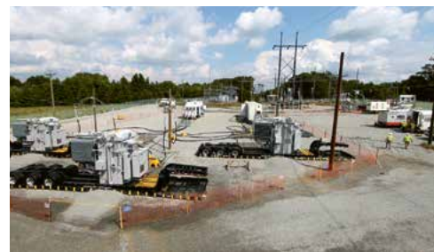
Mobile substation instead of a temporary overhead power line: Dominion Energy breaks new ground in grid renewal with PFISTERER.
