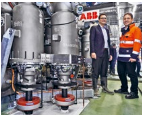
Partners in security of supply: Pascal Müller, General Manager of the new Oerlikon substation (left), and Reto Aeschbach, Sales Manager at PFISTERER SEFAG AG (right), are delighted with the successful fusion of environmentally friendly technologies: dry-insulated HV-CONNEX cable terminations from PFISTERER in use with an eco-gas-insulated HV switchgear from ABB (to the left of the image).
