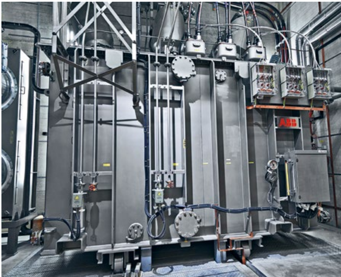
Efficient use of space: 50-MVA power transformer from ABB installed in one of the underground transformer cells at the new Oerlikon substation, connected to heat exchangers for energy-saving use of heat and fitted with compact connection and monitoring solutions from PFISTERER
