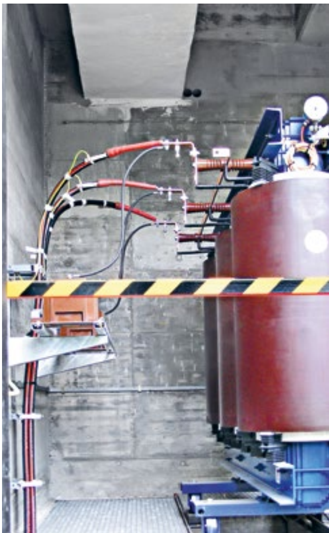
Figure 5: Voltage tests on cast-resin transformers present a very high risk of interference fields – especially if it is only possible to make contact with the busbars being tested from the side, as is the case here.
