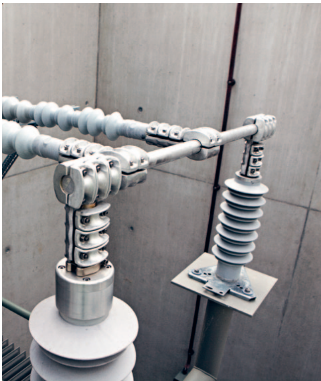
PFISTERER custom solution for connecting the new transformers in the Verbois substation: Connection from the transformer implementation to the energy arrester with integrated surge protection technology.
