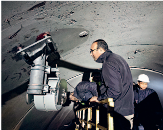
Managers of the railway association TCDD and the railway construction company CRCC inspect the installation of a TENSOREX C+.
