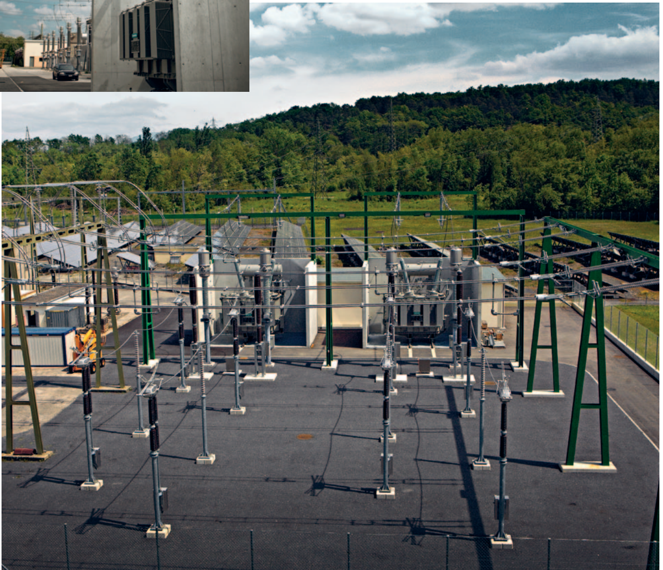
PFISTERER terminal chains and FSK clamps were used for connecting the new transformers to the current transformer (small image on the left).
