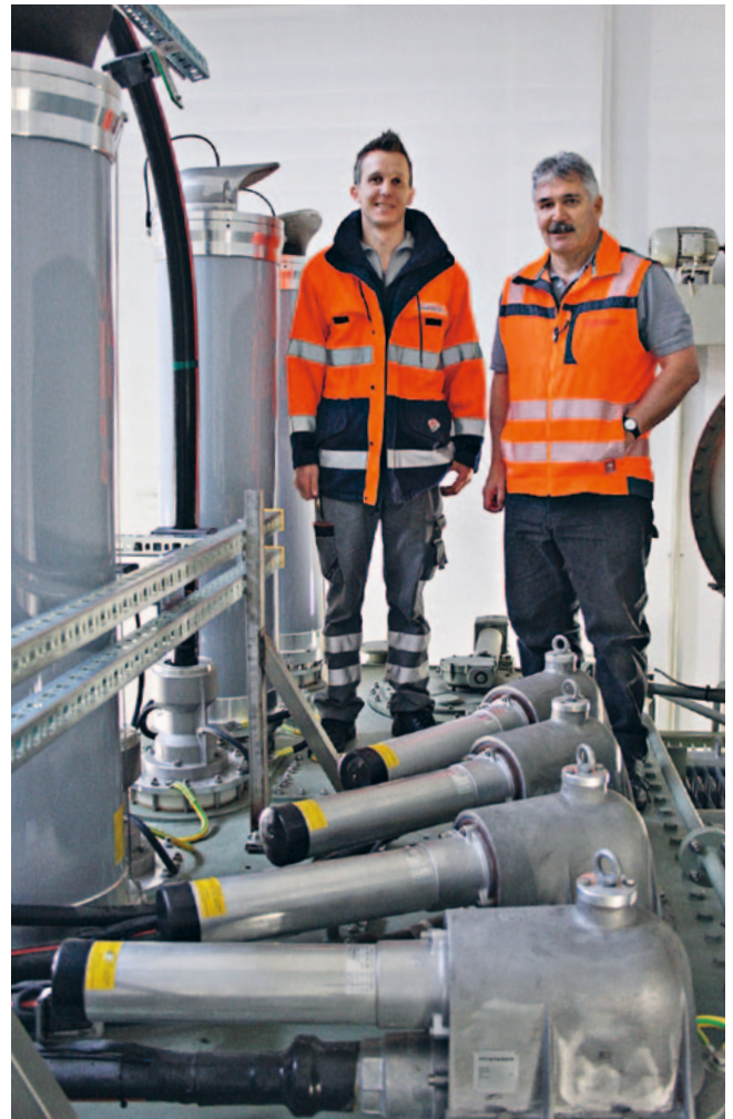
Easy to install meets installation experience: The PFISTERER technicians Peter Barmettler (left) and Heiri Bissig (right) installed four of a total of eight CONNEX HV surge arresters 5-S in nine hours total. Foreground of image: With CONNEX multi-angle connection pieces, medium voltage cables and arresters can be installed directly next to each other and also set up horizontally. This not only saves space, it can also guide the critical field lines closely alongside the system as to maintain the system thresholds.
