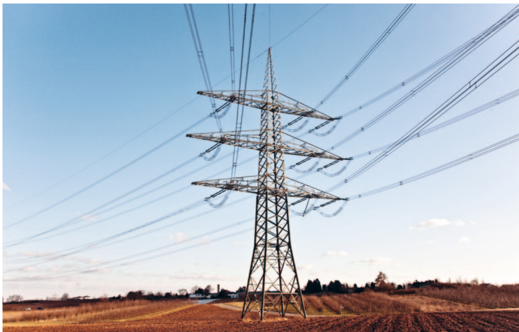
The more space overhead corridors require, the more laborious the permit procedures. An advanced alternative is space-saving compact cables (see illustrations on page 10 and 11).
