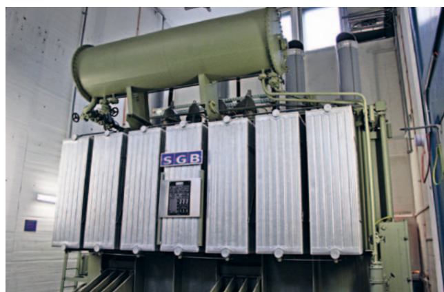
Unique surge protection for multiple advantageous retrofit applications: Four dry, pluggable CONNEX surge arresters, size 5-S, in use on a 25-MVA regulating transformer that is equipped with 110-kV and 16-kV cable connections and therefore completely converted to the CONNEX connection system.
