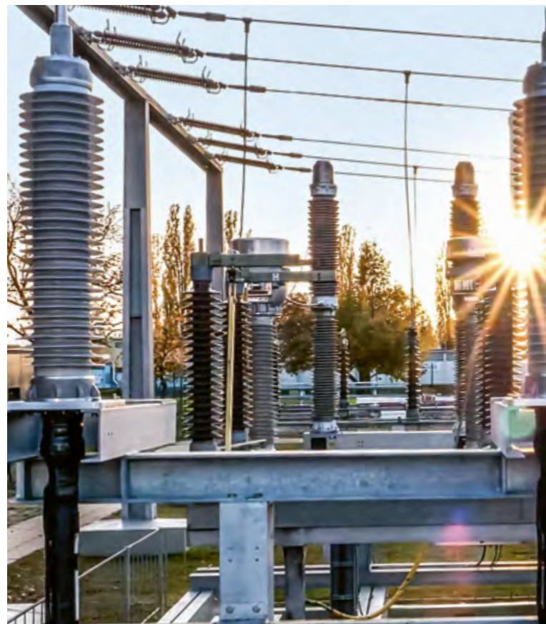
At the substation in Graz, maintenance-free operation of the environmentally safe terminations means less monitoring is required from now on.
