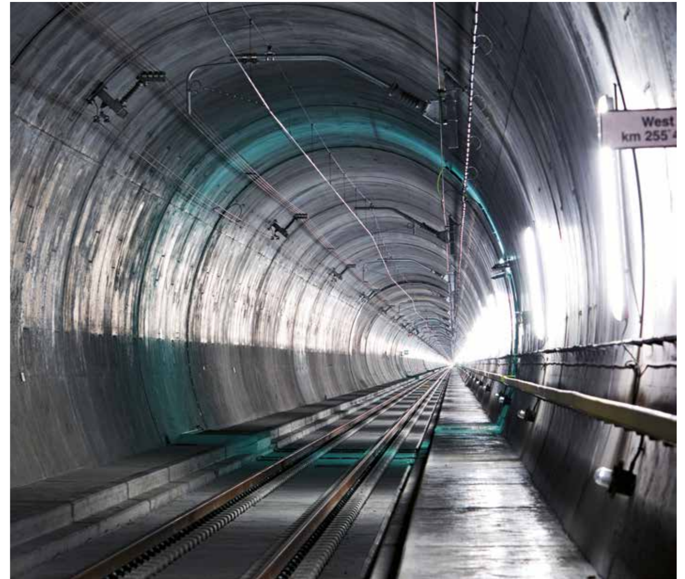
For reliable use under hard conditions: PFISTERER supplied time-tested and custom-built safety equipment for the new Gotthard Base Tunnel, which counts as the world's longest railway tunnel to date at 57 km total length. [© AlpTransit Gotthard AG]
