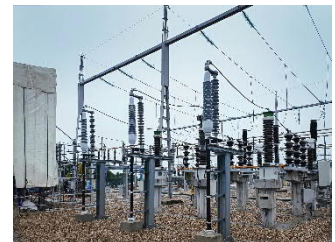
i-DE Redes Eléctricas Inteligentes is using the EST retrofit solution from PFISTERER to replace old porcelain terminations.
